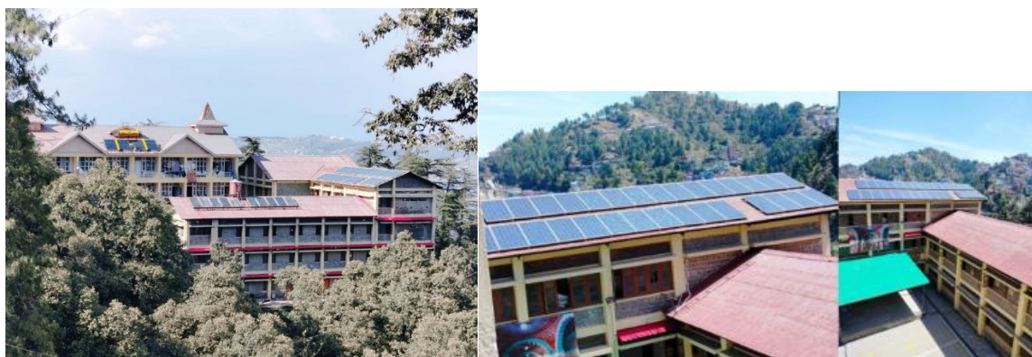
Solar panels installed on the hostel building.
