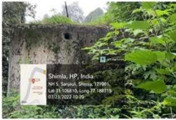
Rain Water Harvesting Tank
